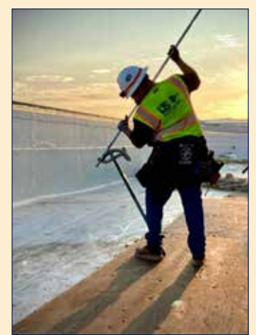
IBEW Local #11 member Charly Xicara with DSE Electric on the rooftop of the NFL Headquarters in Inglewood.
